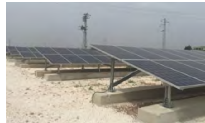
Turkey's largest solar powered irrigation system
